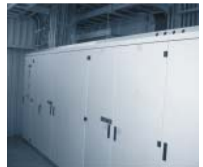
Drive IT ACS 1000 controlling the SAG mill at Agnico-Eagle's LaRonde mine.
