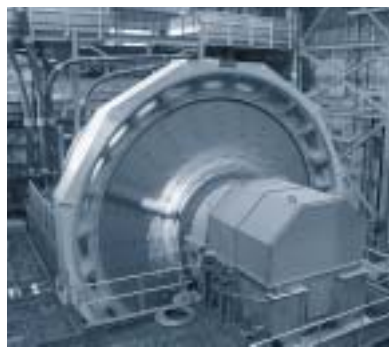
View of the SAG mill (3360 kW).
