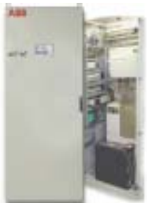
Emissions Monitoring System
