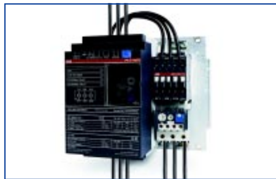
A typical "Inside Delta" combination as a replacement for a Y/D-starter
