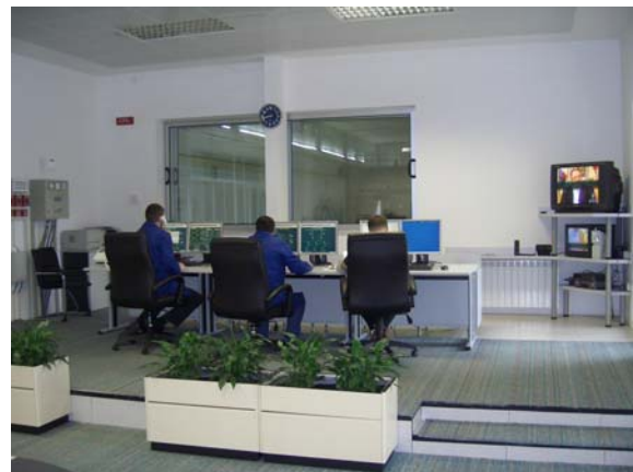
Control room with the 800xA System
