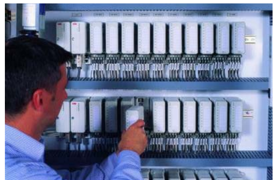
Redundant controller AC 870P (top right) and Remote I/O of System 800xA (below)
