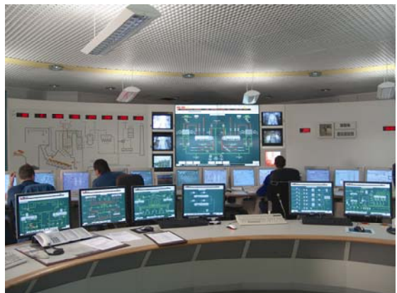
Modern power plant control room based on System 800xA
