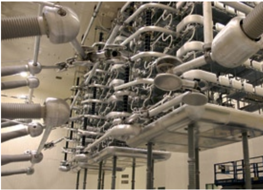
Valve hall at Sylmar East.
