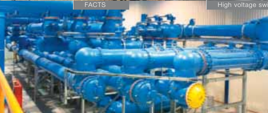
High voltage switchgear
