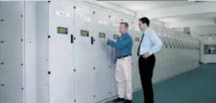
Medium voltage switchgear
