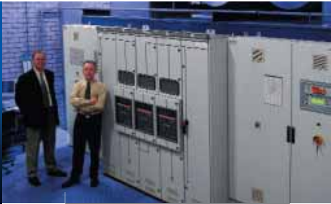
Low voltage switchgear
