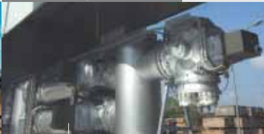
High voltage switchgear
