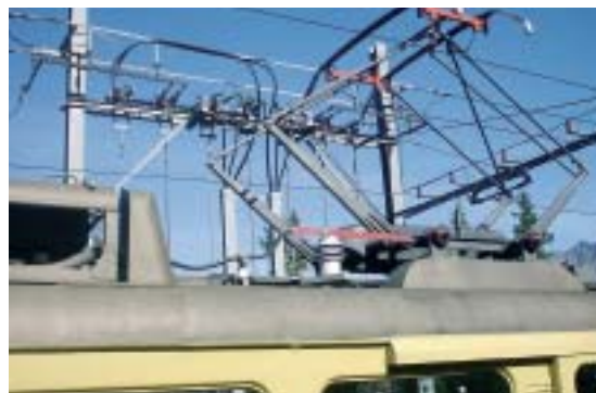
Figure 13: Example of an arrester installation on a railway.
