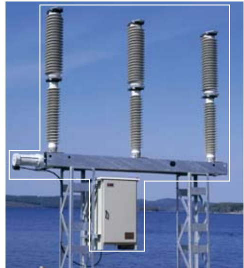
For best availability the whole circuit breaker system is continuously supervised
