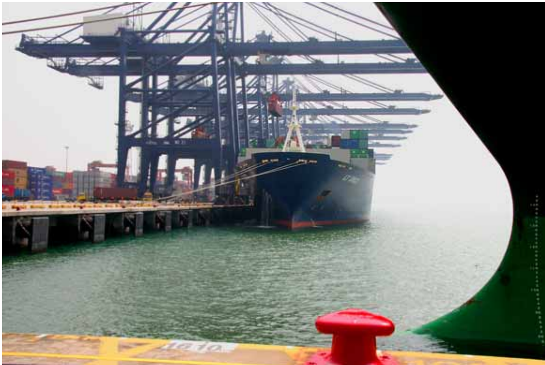
ABB motors power the STS (ship to shore) cranes in the Port of Miami. Each crane contains 4-5 ABB motors.
