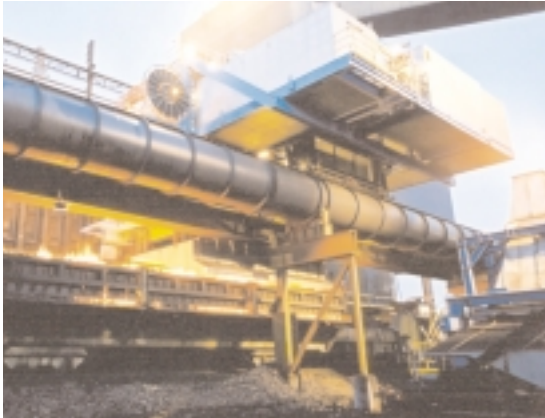
In the early 1990s, ABB installed three MasterPiece 200/1, replacing old relay technology at the coking plant.
