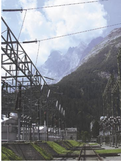
The primary equipment of the Innertkirchen 220 kV substation will remain in service also after the retrofit.
